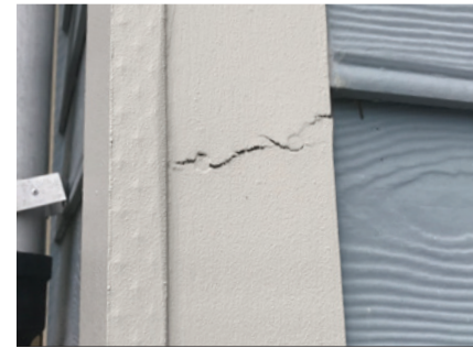
FIBER CEMENT Cracks open the way for water infiltration.
