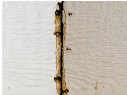
ENGINEERED WOOD Unsealed ends? Rot is coming.
