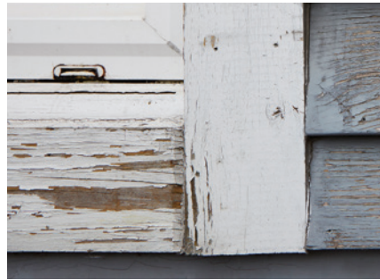
PAINTED WOOD Paint needs constant repainting.
