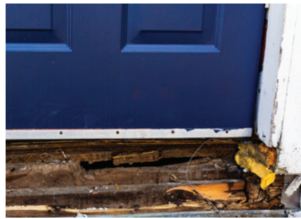
PAINTED WOOD Moisture cycles destroy wood.
